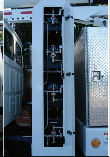
CNG FUEL STORAGE ENCLOSURE
